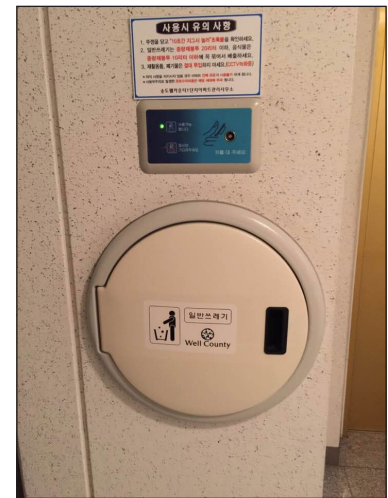
Fig. 5: The door in the staircase opening onto a pipe, which transports the domestic garbage on to the waste disposal plant.
